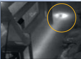
Underground steam leaks
